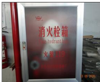
Photo of fire safety equipment Fire hydrant.JPG
