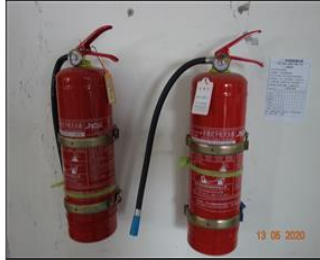
Photo of fire safety equipment Fire extinguishers.JPG
