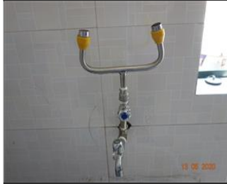
Photo first aid facilities Eye wash system.JPG
