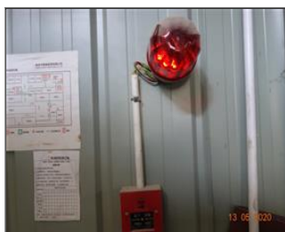
Photo of fire safety equipment Fire alarm.JPG
